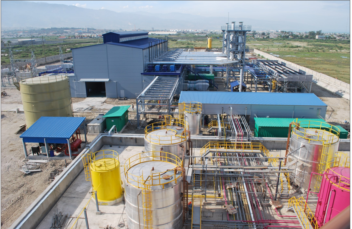
Heavy Fuel Oil Power Station—Haiti
